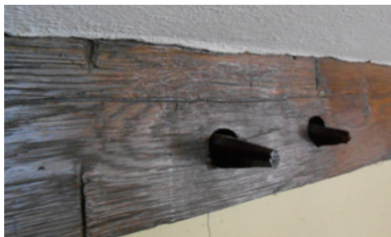
Original hand-hewn beams are held together by wooden pegs in the attic of the farmhouse
